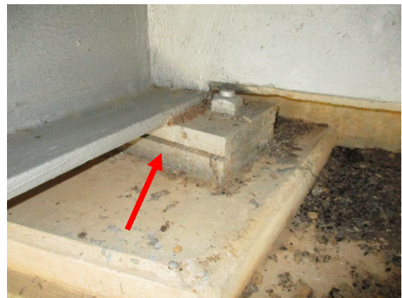
Photo 6. LBP on Gray Bearing Plates.
