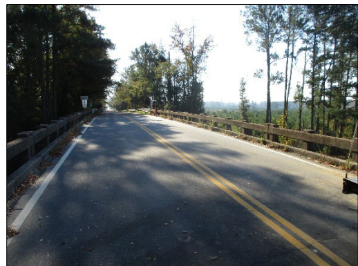
Photo 1 – US 21 (Frampton Rd.) Bridge over CSX Railroad, Hampton and Beaufort Counties, SC.
